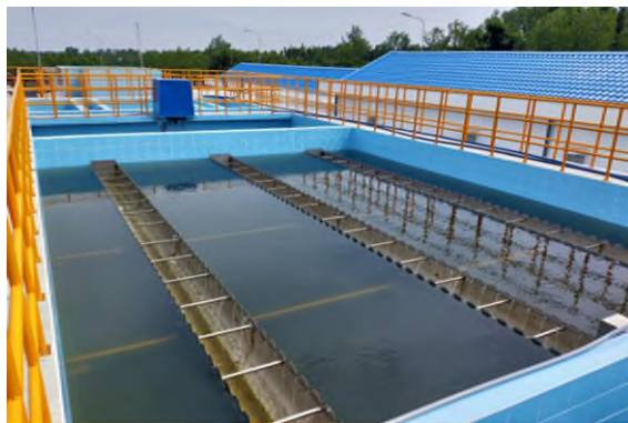
Darco Ba Lai Water Treatment Plant
